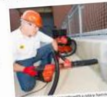
Worker drilling into concrete with a jackhammer equipped with a shroud and vacuum collection system.
